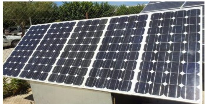
Fig.3. Photovoltaic panels of 80 Wp.
