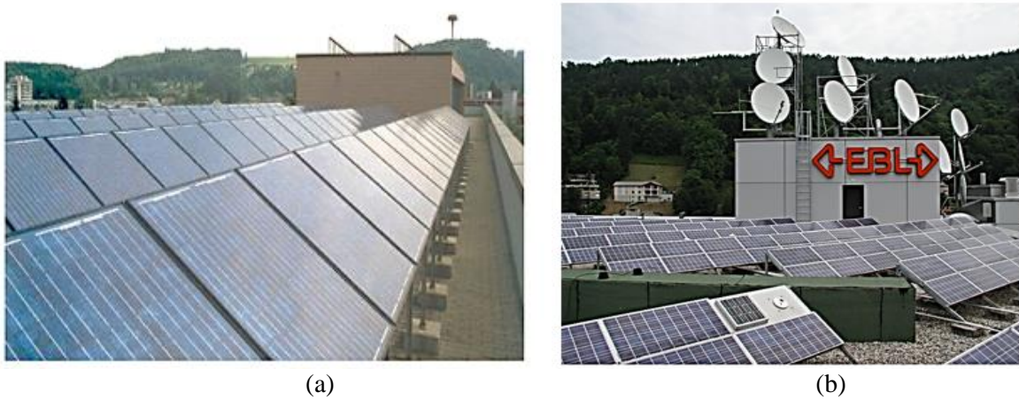
Fig. 4. (a) PV plant Localnet, Burgdorf (Switzerland) (b) PV plant EBL Liestal (Switzerland) [14].
